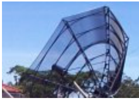
A satellite dish installation at Egerton University. It is still very expensive for educational Institutions to acquire Internet connectivity commercially.
