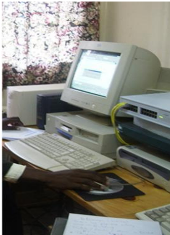
The Server, Router, Switch and UPS supplied to Western College – Kakamega (WECO) by KENET
