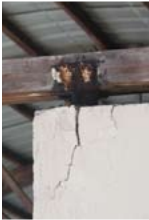
HAY NECESIDAD DE CAMBIAR EL TECHO ROOF WILL NEED TO BE REPLACED AS THE SUPPORT BRACKETS ARE RUSTED
